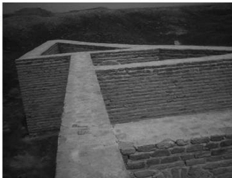
FIG 2: DAMAGE DUE TO UNSCIENTIFIC MAINTENANCE, AND USING EXTRANEOUS MATERIAL IN MAINTENANCE SUCH AS CEMENT, GRAVEL, AND MODERN BRICKS
